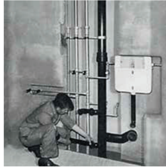
↑ Introducing the first concealed cistern in 1964
